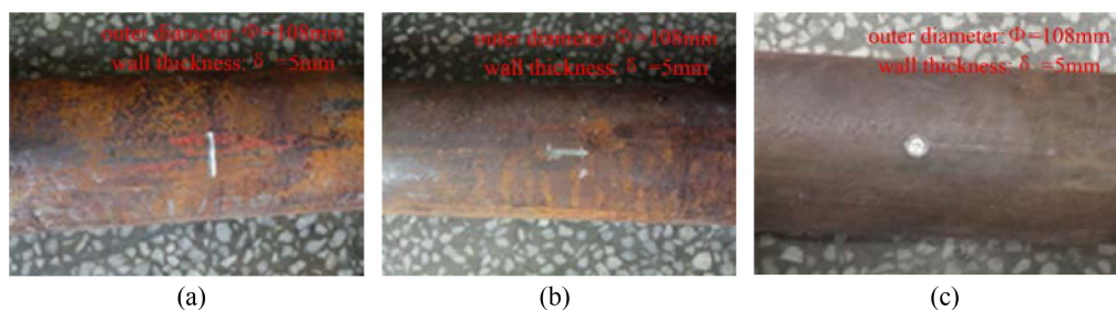
Fig. 13. (Color online) Three typical types of pipeline defects: (a) Circumferential groove; (b) Axial groove; (c) radial circular hole
